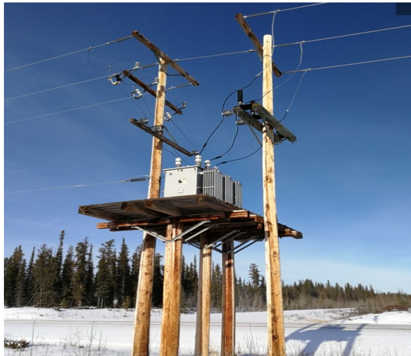
Figure 3-7: Typical Pole Mounted Transformer Station
