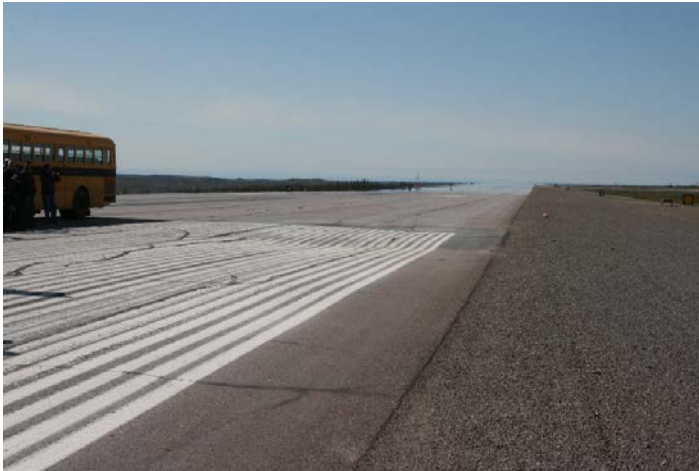
Photo 1. Sinkhole on runway (June 2011).
