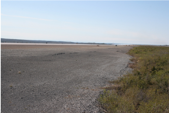
Photo 4. Tension cracks along the runway embankment looking West (June 2011).
