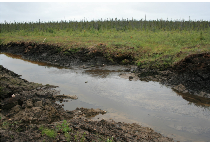
Photo 6. Water ponding in diversion ditch East of Taxiway E (July 2015).
