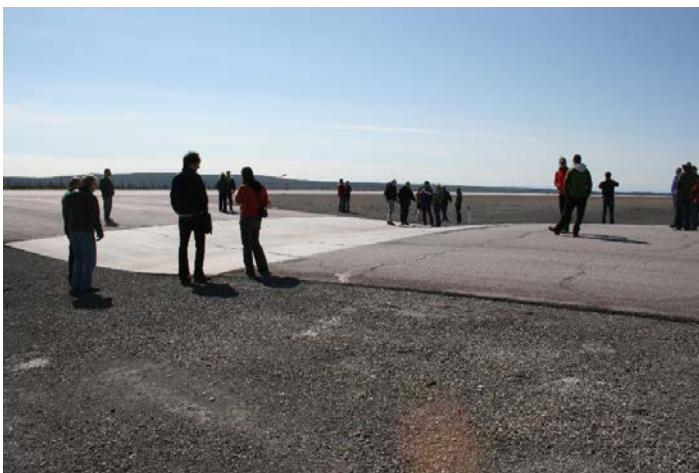
Photo 3. Subsidence on Taxiway E (June 2011).
