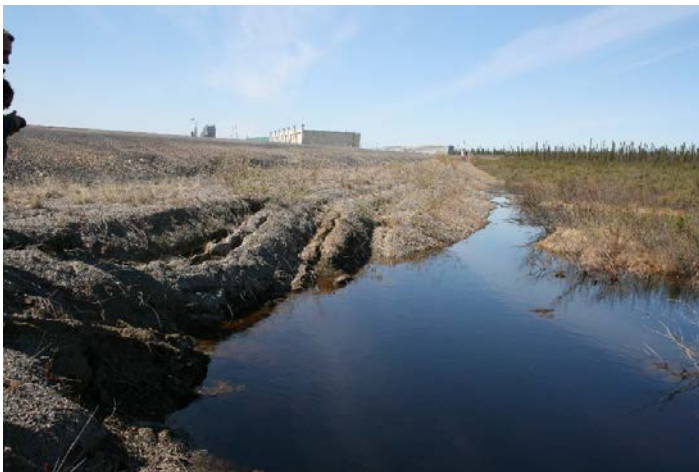
Photo 2. Sloughing and water ponding at toe of Taxiway E embankment looking North (June 2011).
