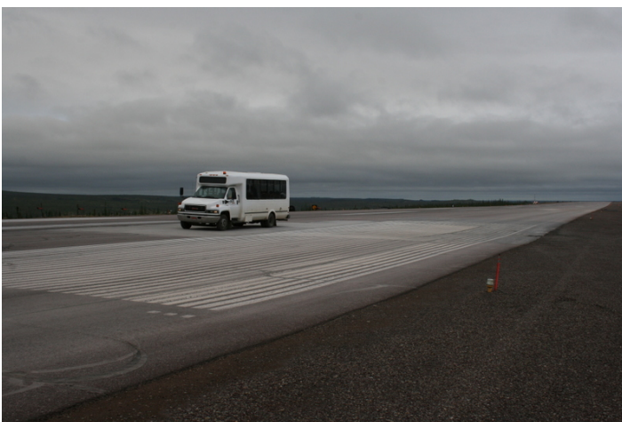
Photo 15. Fixed sinkhole (see Photo 1; Report, Figure 2-6) on runway (July 2011).
