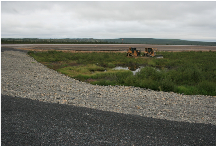
Photo 5. Water ponding in diversion ditch West of Taxiway E looking towards the runway (July 2015).
