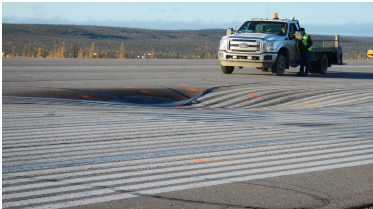
Figure 2-6. Runway 06/24 subsidence (Tetra Tech EBA, 2013).
