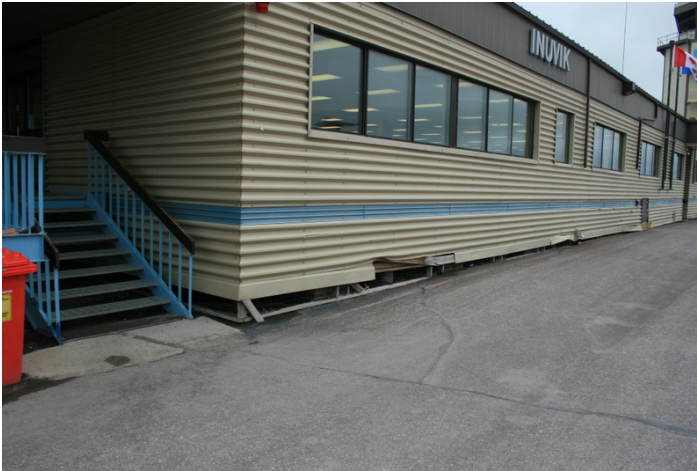
Photo 16. Settlements under air terminal building (July 2015)
