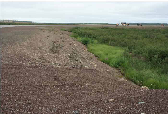
Photo 14. Embankment of Taxiway B sloughing, looking towards Taxiway D (July 2015)
