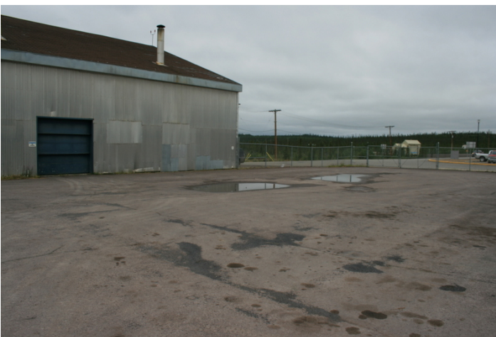
Photo 18. Water ponding on apron between air terminal building and hangar, looking north (July 2015).
