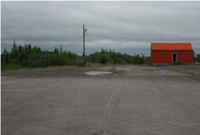
Photo 19. Northeast end of apron showing differential settlements and water ponding (July 2015).
