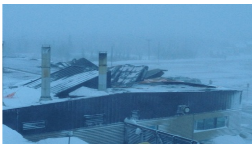
Figure 8: Blizzard Damage to Inuvik Airport Roof - January 2012 (Source: GNWT, MACA)
